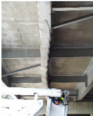
View of Beam BEFORE Repair
